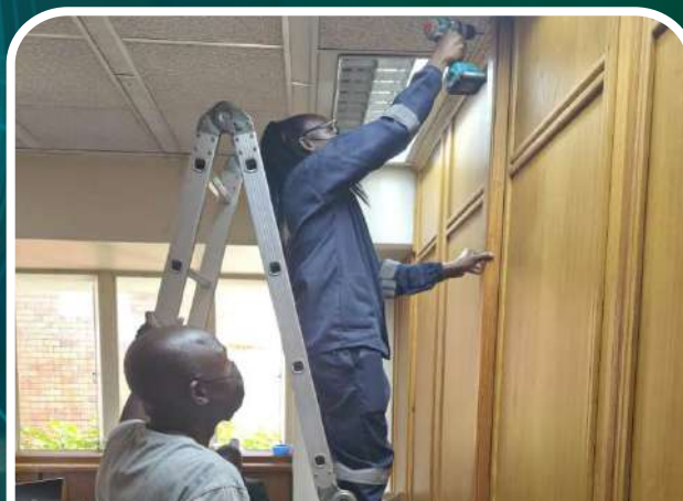
NPAZ IT Technical Support Specialists Tonderai Mudyiwanyama (left) and Faustina Mtisi (right) carry out CAT 6 cable installations on the 6th Floor of the NPAZ Head Office in Harare, recently.
